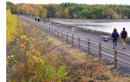
RAIL TRAIL WITH INTEGRATED PROTECTIONS AND DRAINAGE Ashokan Rail Trail, West Hurley, New York
