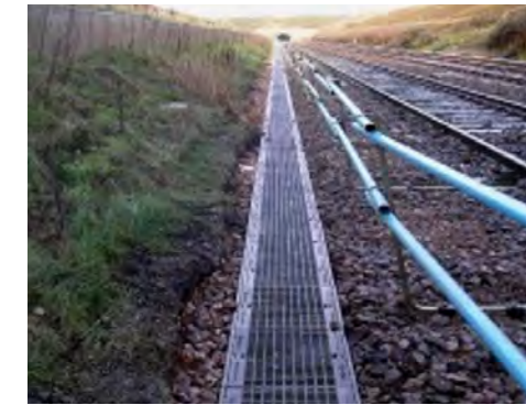
IMPROVED PERCOLATION ALONG RAILWAY LINE Severn Tunnel East, UK
